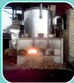
Thermic Fluid Boiler
